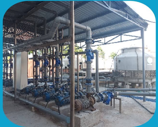
High Efficiency Pumps
