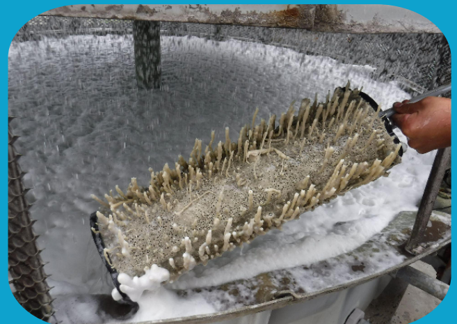
Scale Treatment for Cooling Tower
