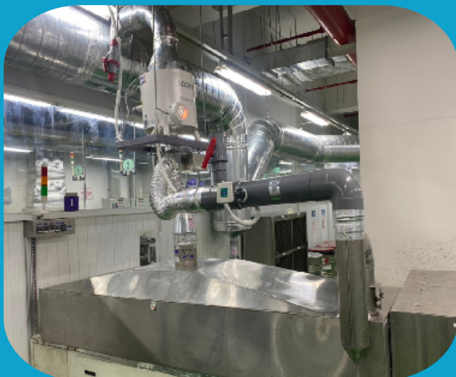
Oil Steam Collection System
